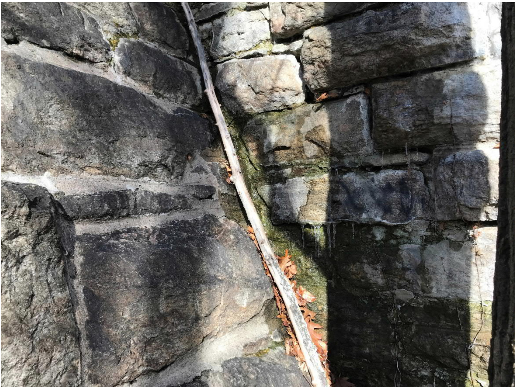
Photo No. 26: Minor seepage/wet spots observed along the downstream joints of the primary spillway wing walls and the masonry dam on the right side.
