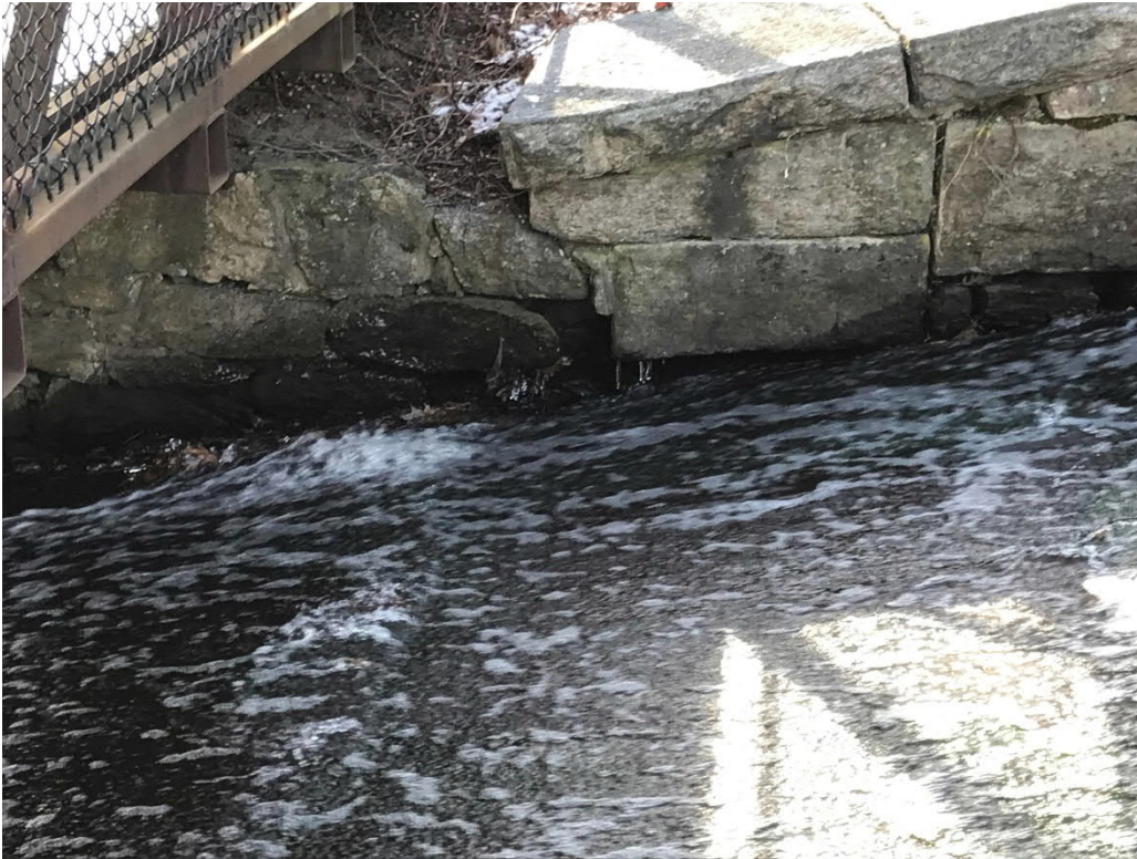
Photo No. 29: Undermining of the primary spillway wing walls along the right side.
