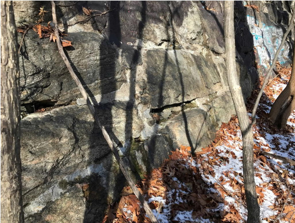
Photo No. 25: Typical chipped/missing mortar along the downstream face of the masonry dam. Note minor seepage/wet spots near the toe of the dam.
