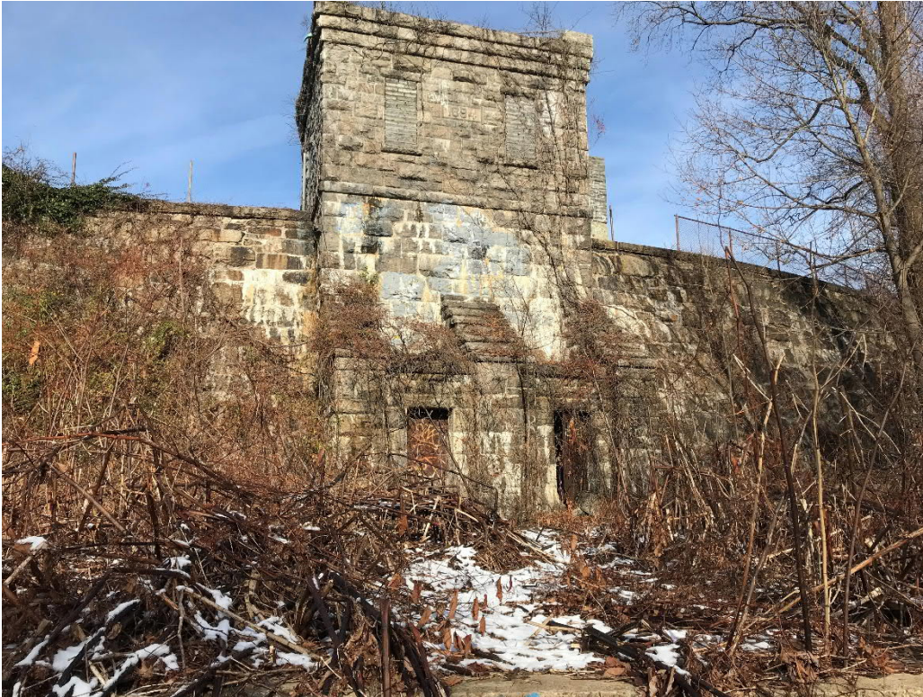
Photo No. 1: Downstream view of the low-level outlet gate house structure located about 150 feet from right side end of masonry dam section.
