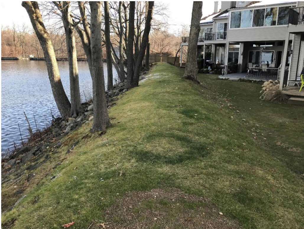
Photo No. 18: View of right earthen dike looking towards the abutment with the right masonry dam. Note the town house complex immediately downstream of the dam.
