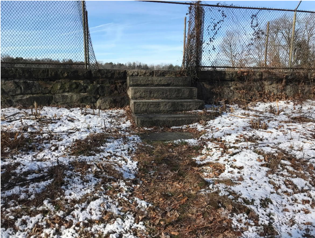
Photo No. 11: View of access stairs to the crest of the masonry dam along the left side. Note the torn/damaged chain link fence.
