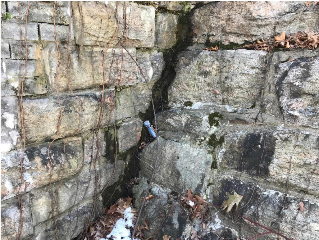
Photo No. 28: Minor seepage/wet spots observed along the downstream joints of the primary spillway wing walls and the masonry dam on the left side.
