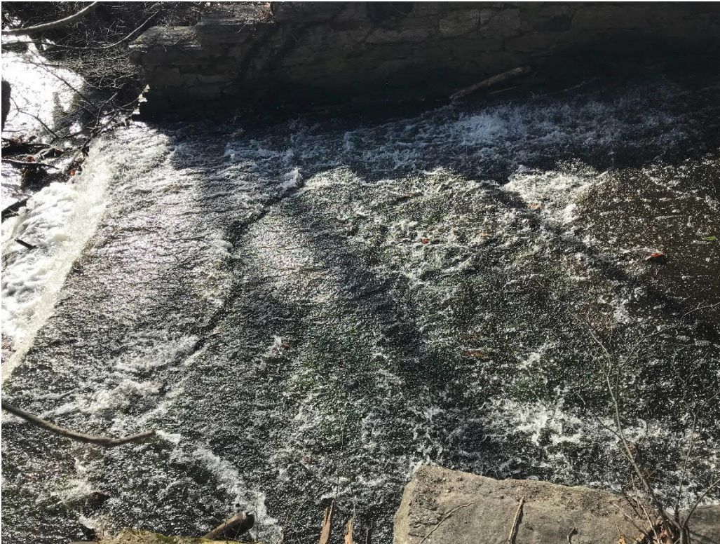
Photo No. 7: View of the downstream end of the primary spillway chute. Note the cracking in the concrete of the chute.
