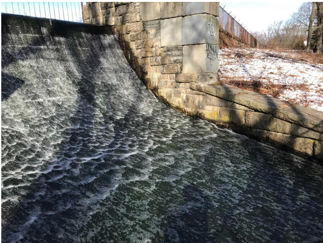
Photo No. 6: View of the primary spillway chute and left spillway wing wall.
