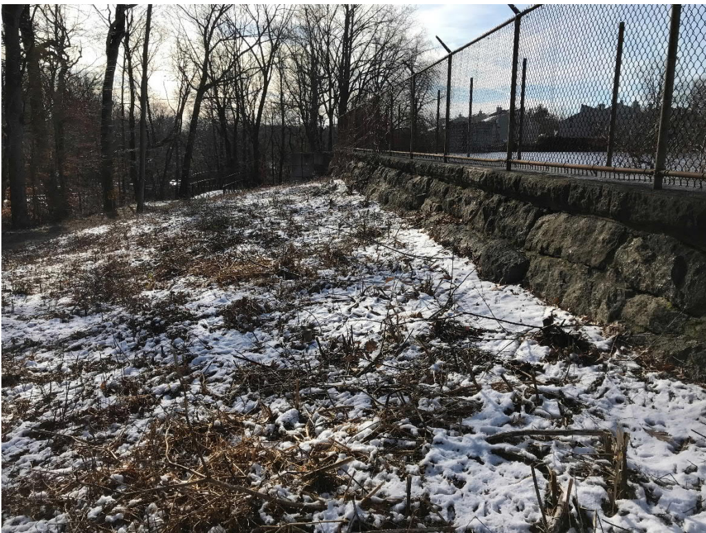
Photo No. 12: View of the masonry dam from the left end looking towards the primary spillway.
