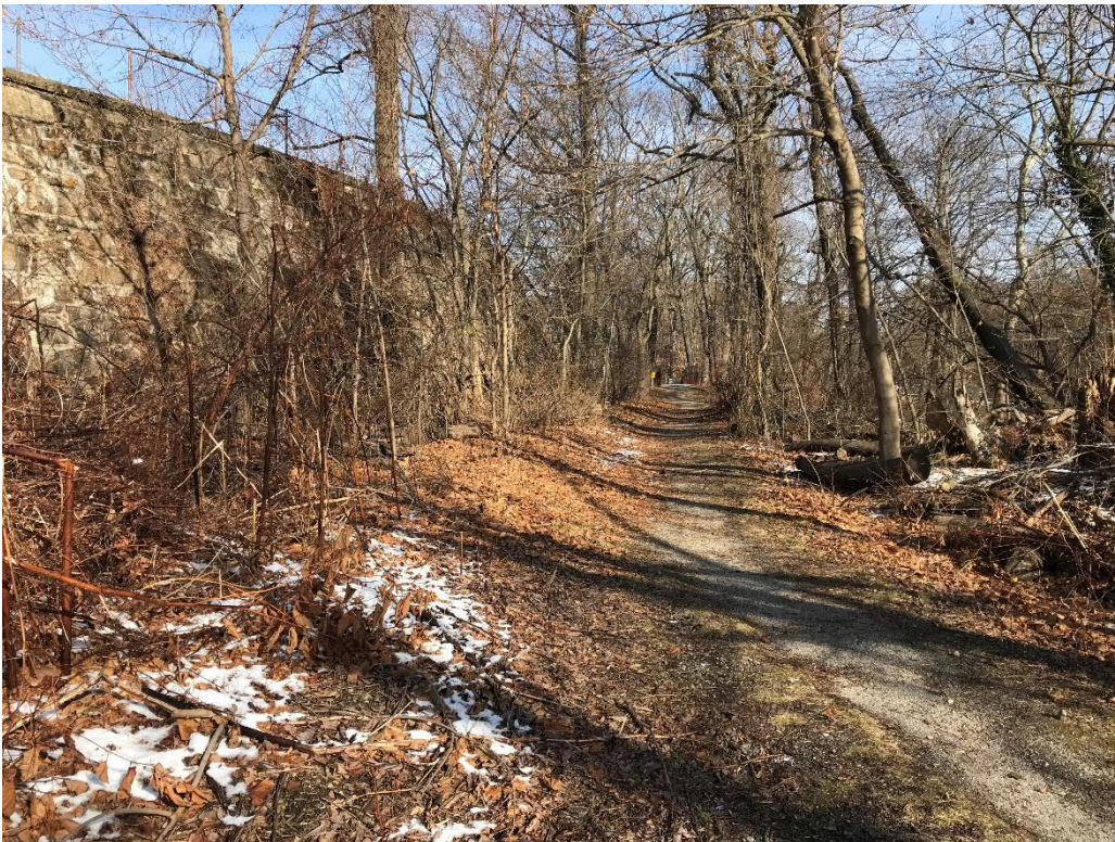
Photo No. 4: Left side of the masonry dam looking from the gate house.
