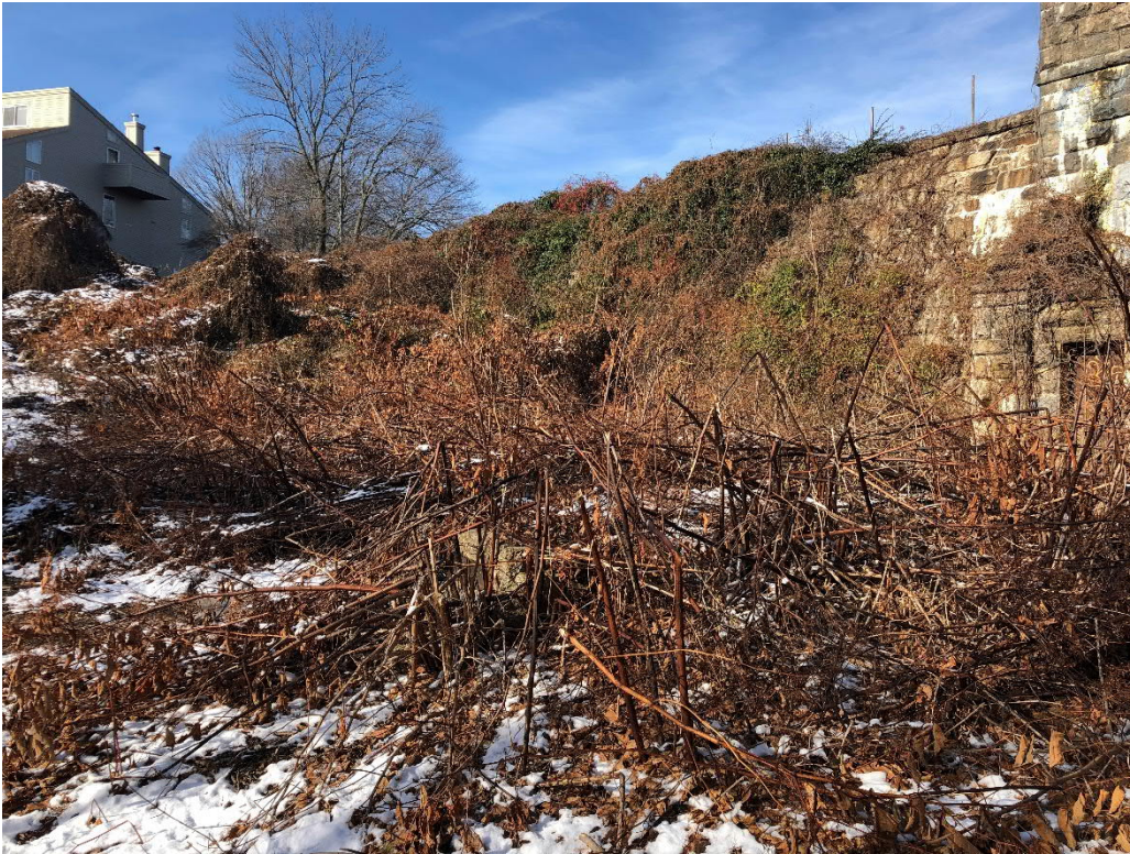
Photo No. 3: Toe of masonry dam along the right side. Note significant vegetation growth.
