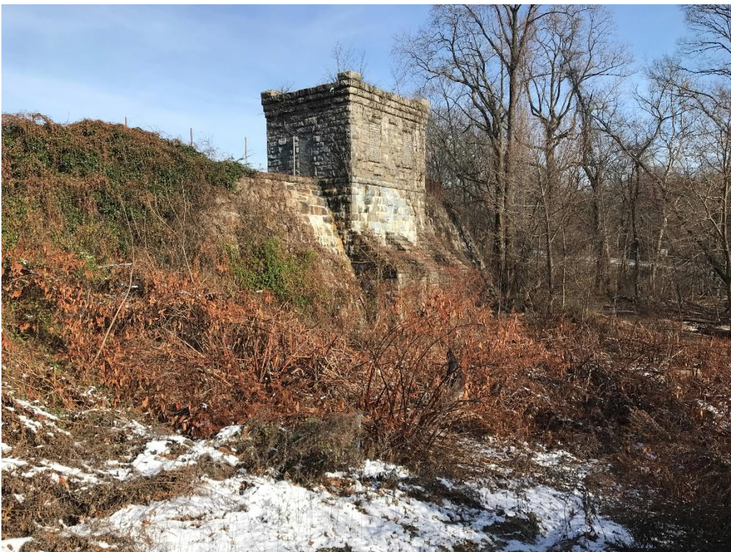
Photo No. 2: Right section of masonry dam looking from downstream. Note significant vegetation growth.
