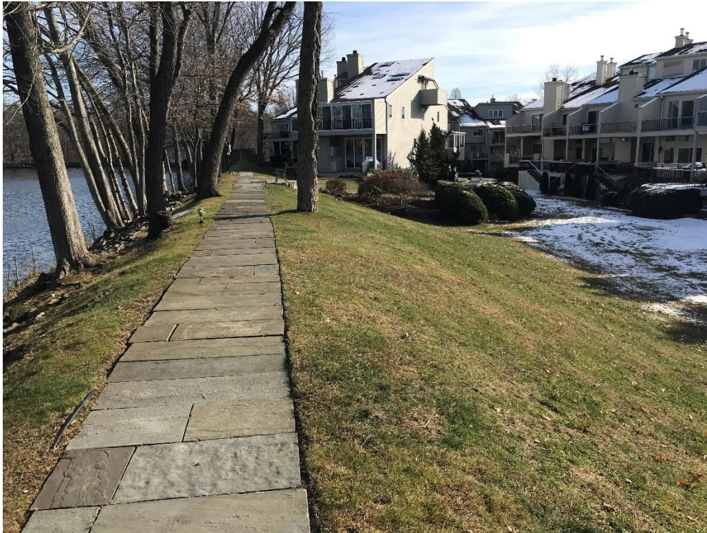
Photo No. 17: View of the right earthen dike looking from the right end of the dam.
