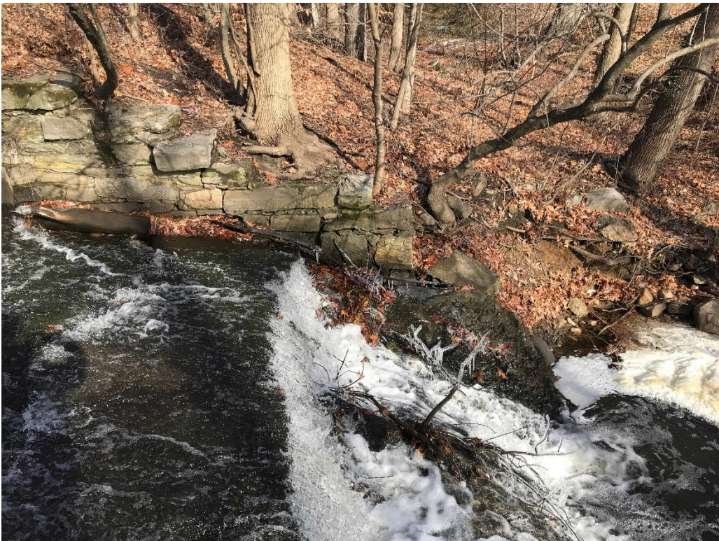
Photo No. 8: View of the downstream end of the primary spillway chute. Note the deterioration and erosion of the concrete.
