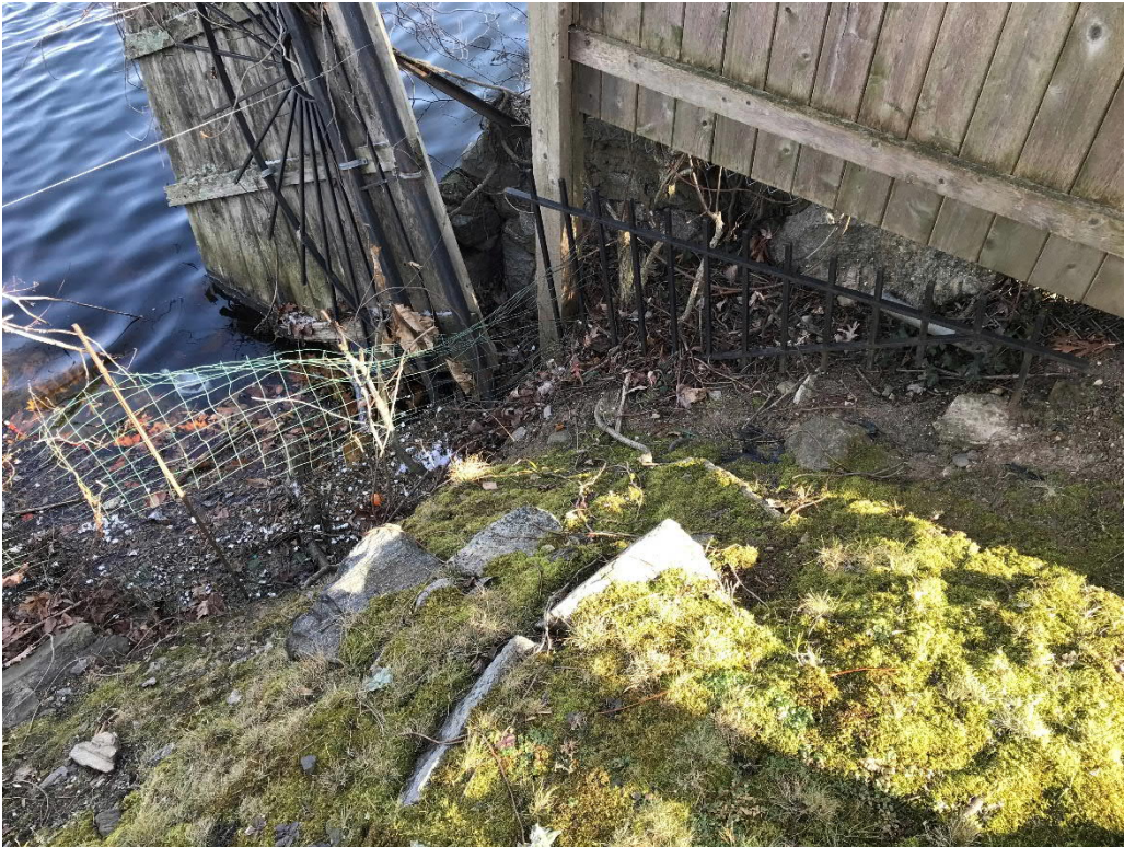
Photo No. 22: Minor erosion observed at the abutment between the masonry dam and the right earthen dike.
