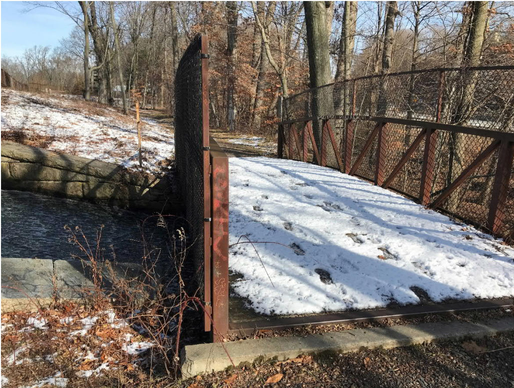
Photo No. 27: View of the pedestrian bridge crossing the primary spillway chute a few feet downstream of the dam.
