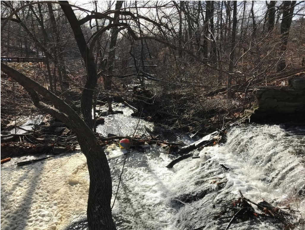
Photo No. 9: View of the downstream plunge pool and discharge channel of the primary spillway.
