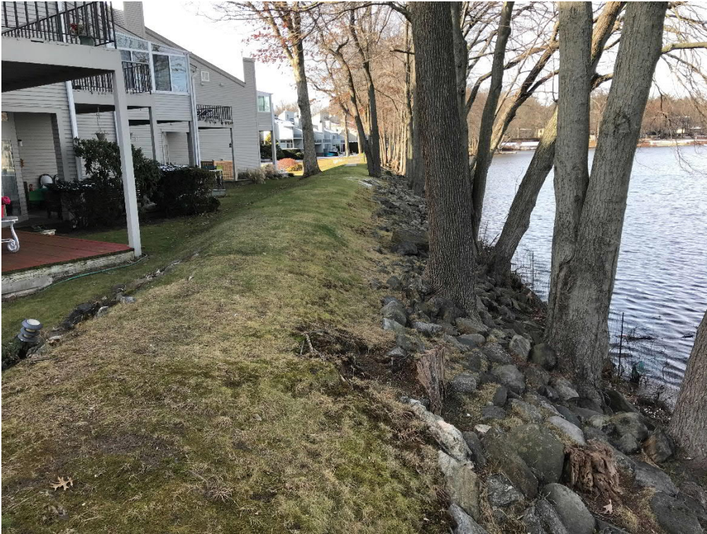
Photo No. 19: View looking across the right earthen dike from the abutment with the right masonry dam. Note trees along the upstream slope and crest.
