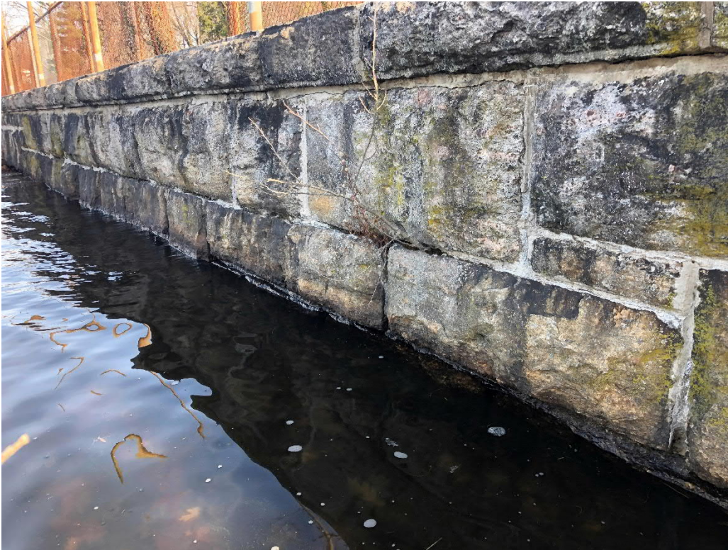
Photo No. 31: Upstream face of the masonry dam left of the primary spillway.
