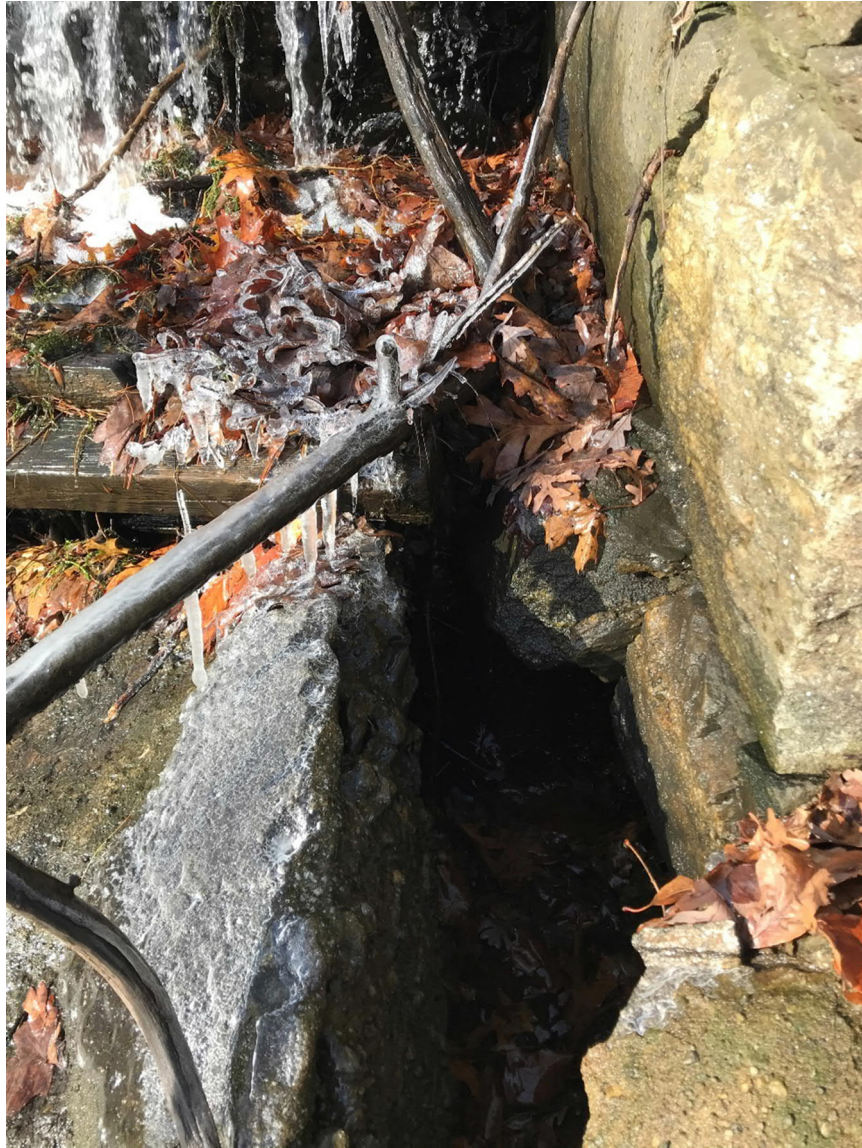
Photo No. 30: Erosion and collapsing of the concrete at the downstream end of the primary spillway chute.
