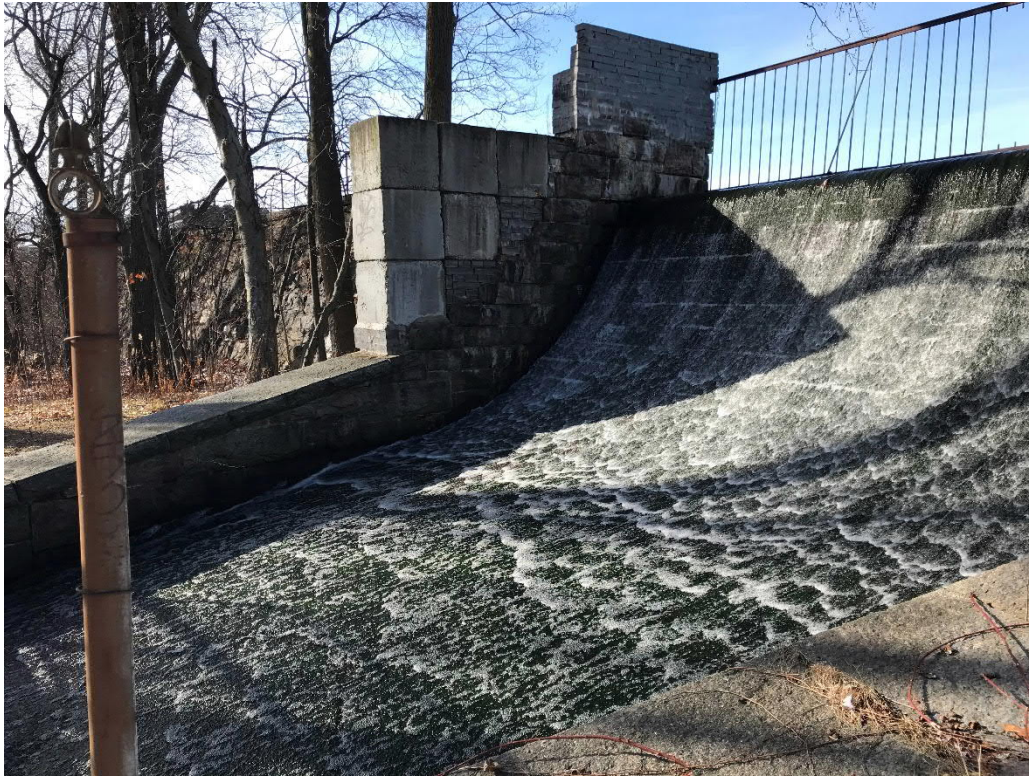
Photo No. 5: View of the primary spillway. Note the wrought iron fence along the crest of the spillway.
