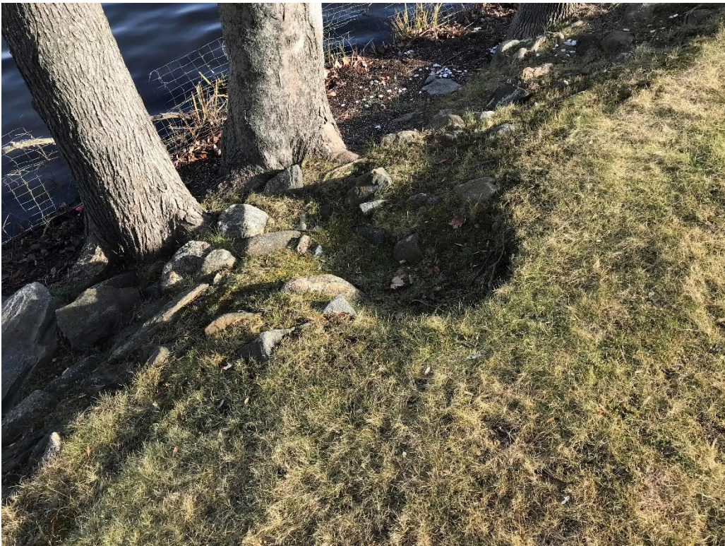
Photo No. 20: Typical erosion/depressions observed along the earthen dike at the right side.
