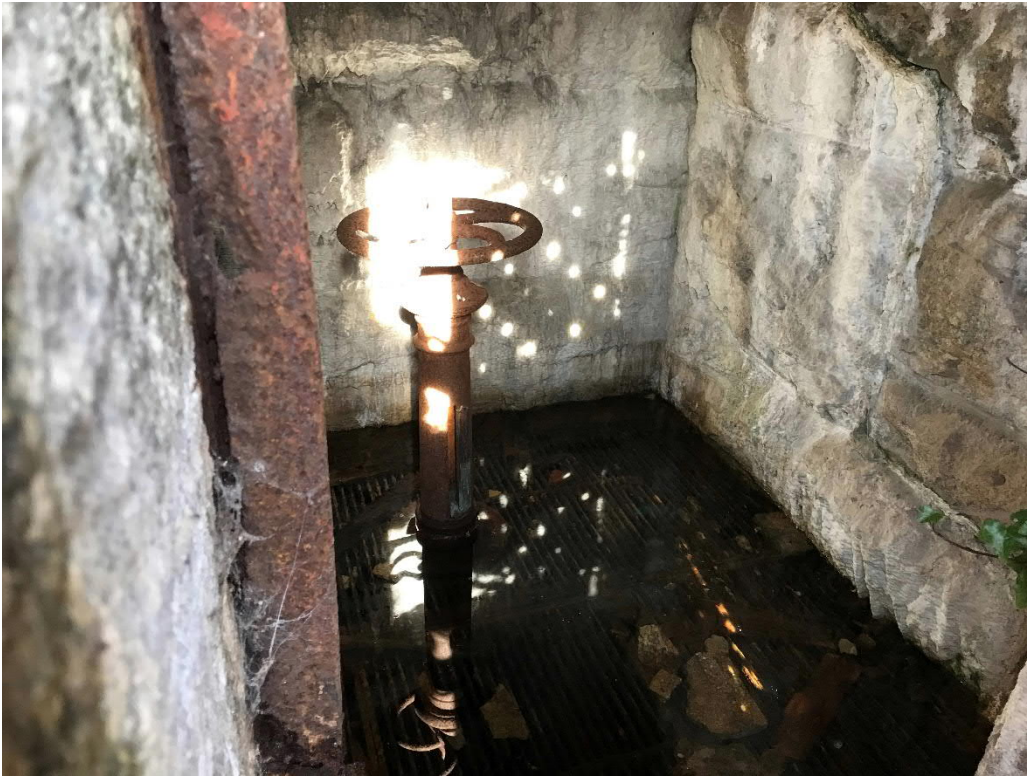
Photo No. 23: View of the valve operator inside the low-level outlet gate house. Valve is inoperable.
