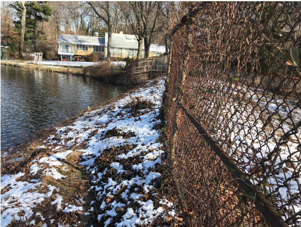
Photo No. 14: View of the upstream slope of the earthen dike at the left side.
