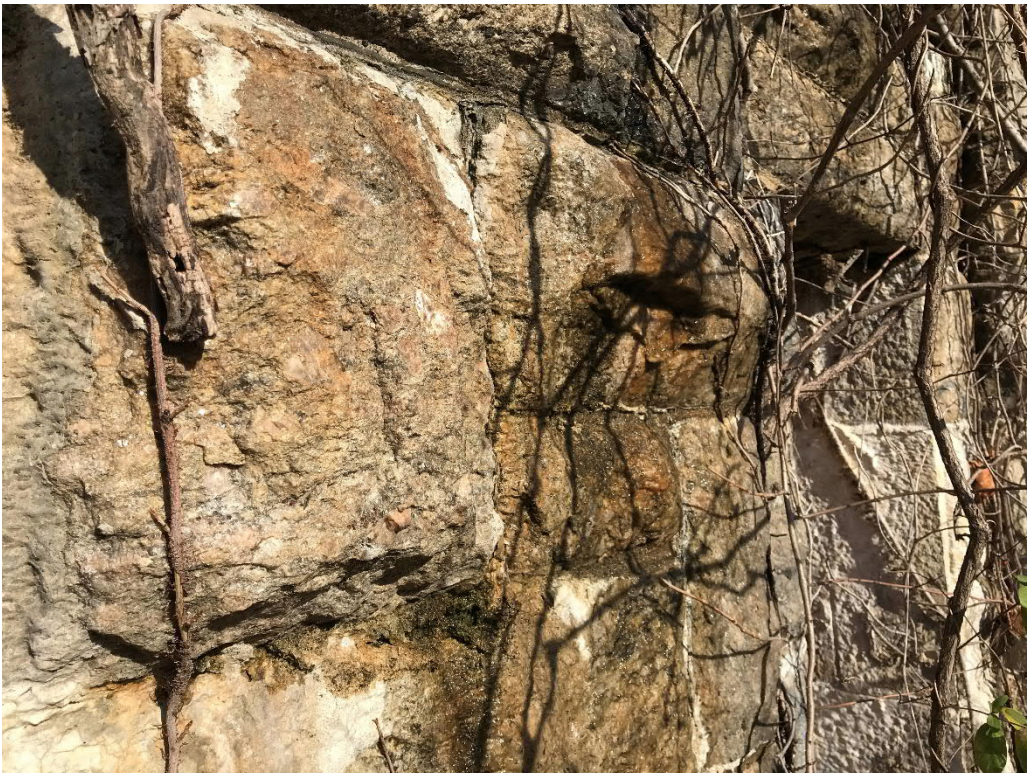
Photo No. 24: Minor seepage observed along the upstream face of the low-level outlet gate house.
